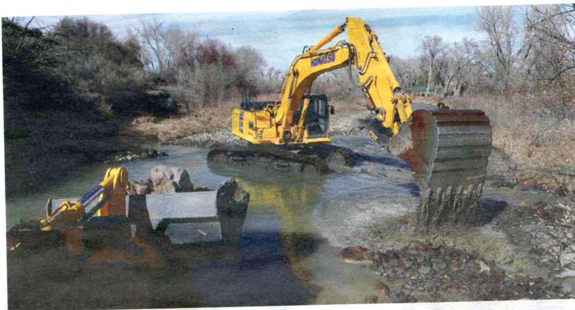
HEAVY EQUIPMENT with Ecological Resource Consultants, Inc. of Evergreen Colo., worked to create new channels, pools and eddies for fish habitat along the Uncompahgre River Tuesday afternoon. About 1,500 feet of the river were reconfigured as designed by the City of Montrose's Uncompahgre River Master Plan. (Photo by William Woody)
